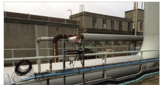
The installed KATflow 170 with stainless steel enclosure at ESSAR Oil
