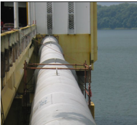
Clamp-on sensors were installed on this existing feeder pipe of a water treatment plant supplying Panama City with water.
